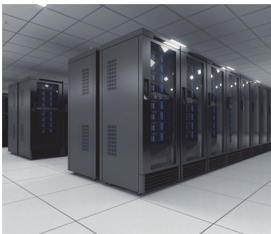
Data centre server room
